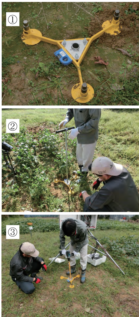
Fig. 4 DDP 設置坑作成の手順①～③. Pictures of drilling a DDP installation hole.
