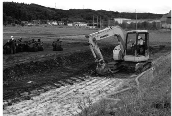
Photo. 15 剥ぎ取り状況. View of peeling.
